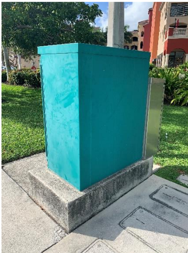
Example of Marco Island Utility Box.
