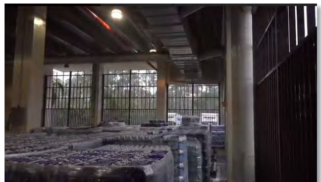
Figure 1: Rain coming into the east bay storage area.
