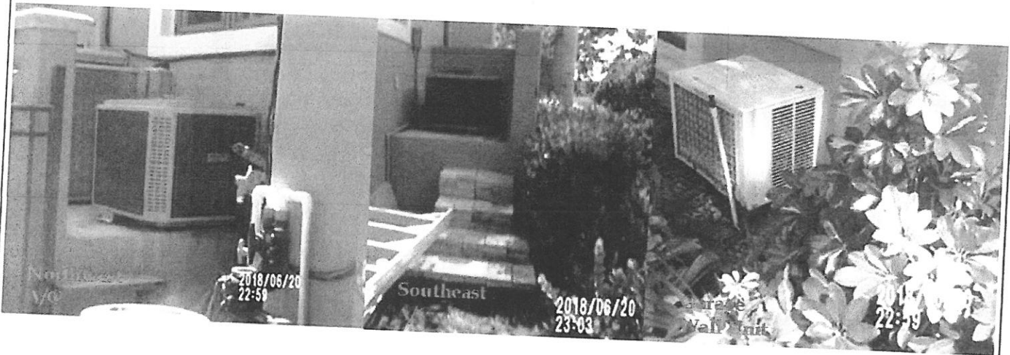
Photo Two Caption A/C Unit View, 06/21/2018
