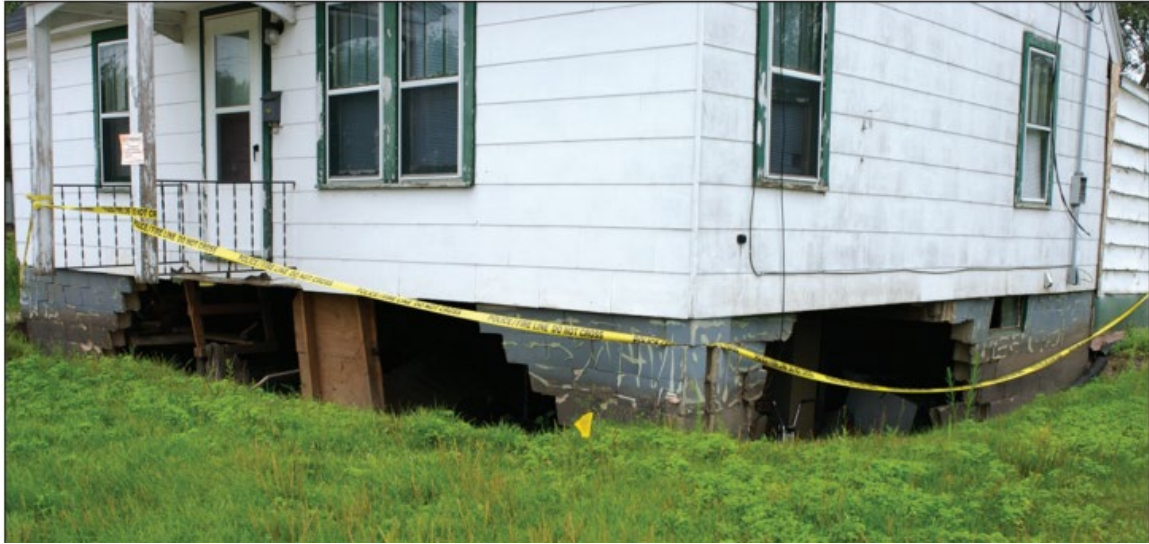
Figure 6: Unreinforced masonry walls of a basement that failed because of the pressure exerted by water and saturated soil
