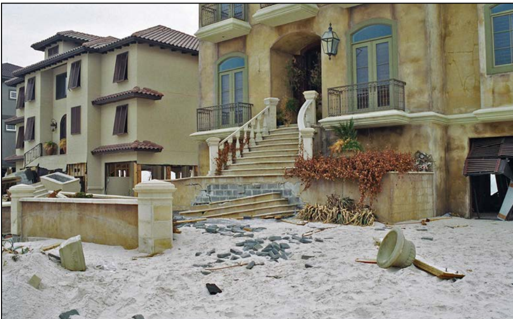
Figure 3: Massive stairs attached to an elevated coastal home, which act as an obstruction
