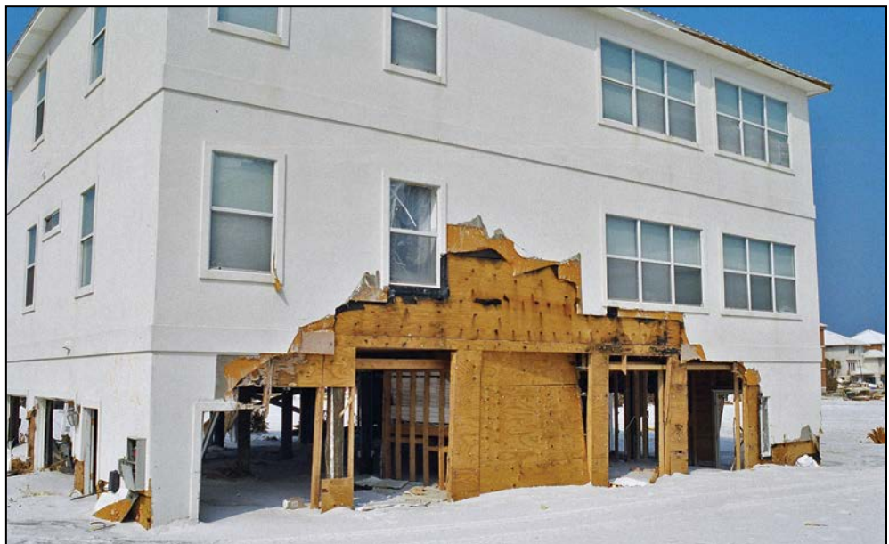
Figure 7: Breakaway wall that did not break away, which led to wave runoff and contributed to flood damage on the side of the elevated building
