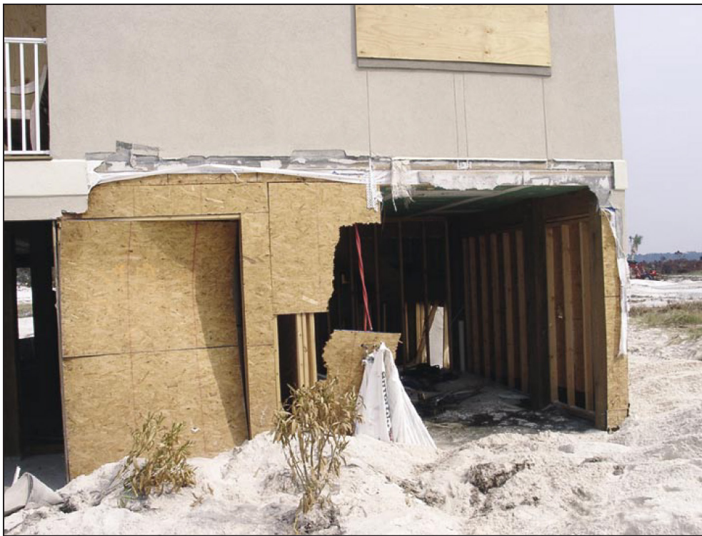
Figure 10: Non-compliant breakaway walls that were nailed over the piles and floor beam, preventing a clean break during Hurricane Ike in 2008 (Gulf Shores, AL)
