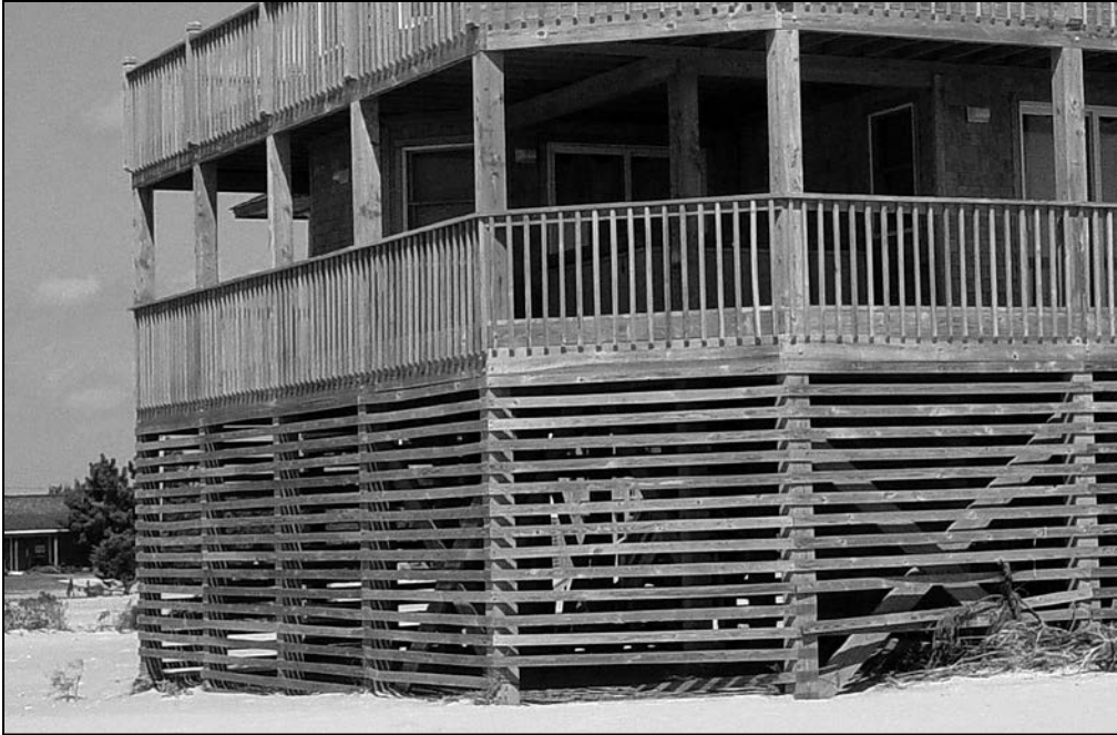
Figure 4: Compliant wood slats installed flat against foundation pilings
