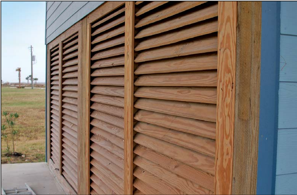
Figure 5: Compliant, fixed, wood louvers installed between pilings
