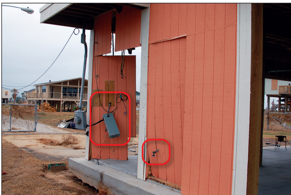
Figure 8: Utilities attached to breakaway walls that may have prevented the walls from breaking away, resulting in additional damage to the structure during Hurricane Ike in 2008 (Galveston Island, TX)
