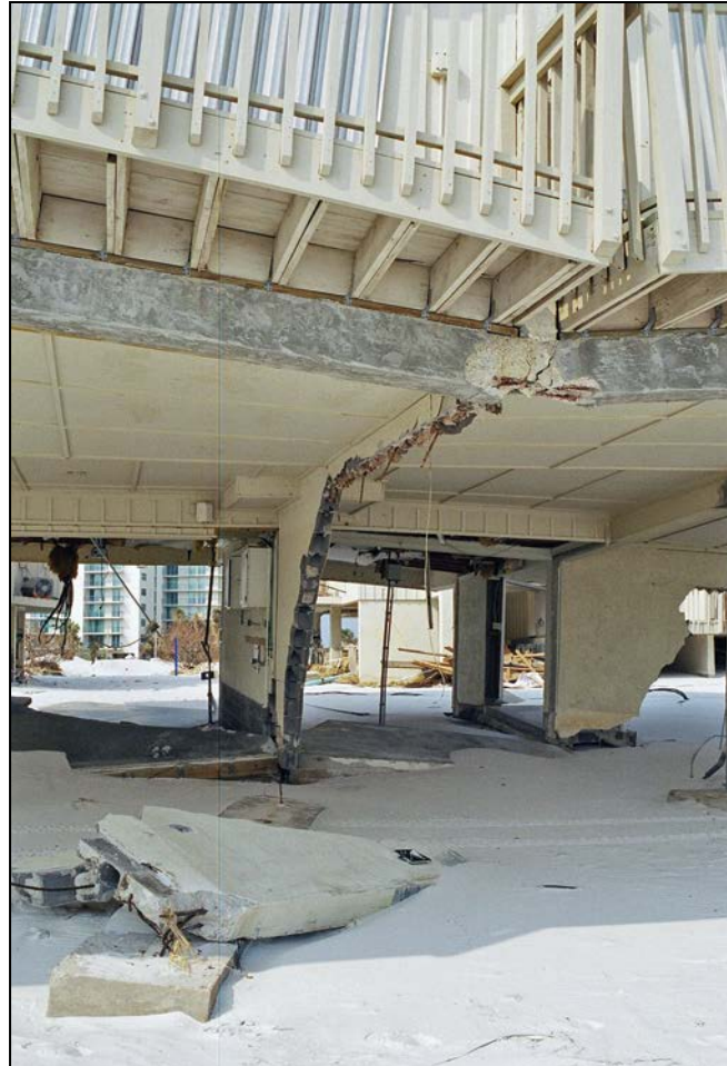
Figure 19: Failure of a shore-perpendicular solid foundation wall that supported a low-rise building, which resulted in failure of the beam and floor system that were supported by the shore-perpendicular wall
