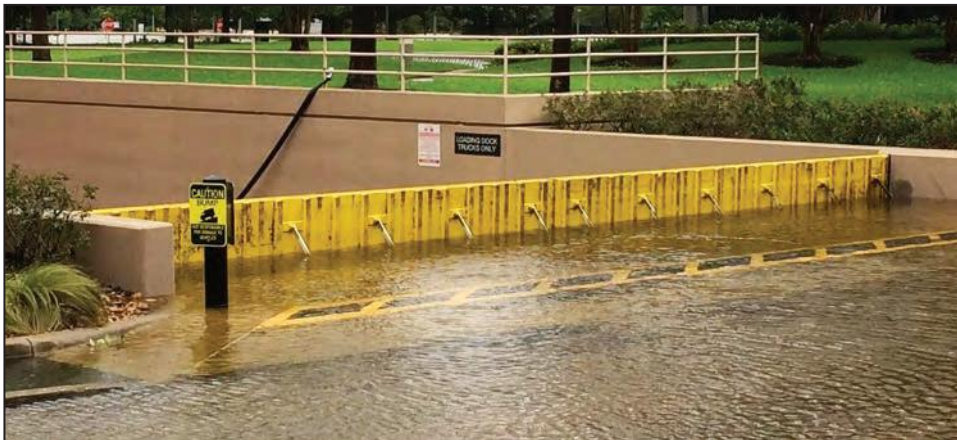
Figure 6: Automatic gate (deploys automatically when triggered by rising floodwater)
