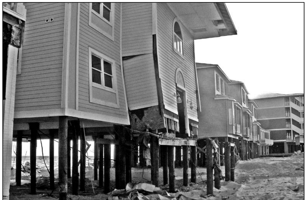
Figure 1: Damage to an elevated building as a result of stairs that did not break away cleanly
