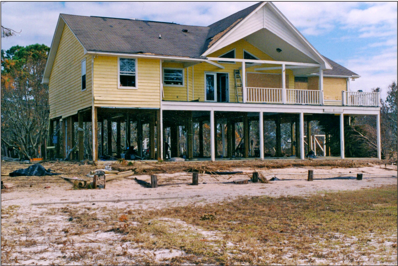
Figure 28: Home elevated above the BFE in Zone AE showing successful failure of breakaway walls.
