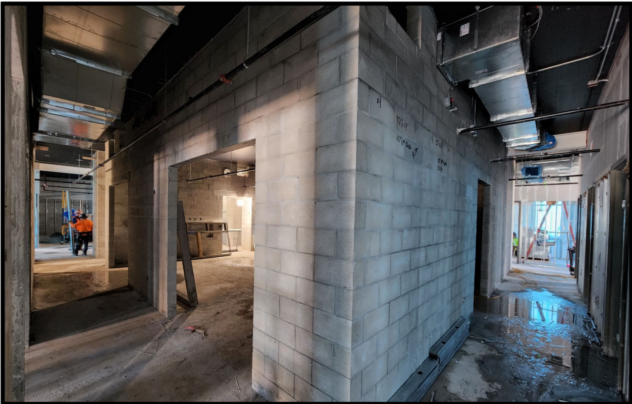
Fire Station 50 – Interior (Bunkrooms and Fitness Area)
