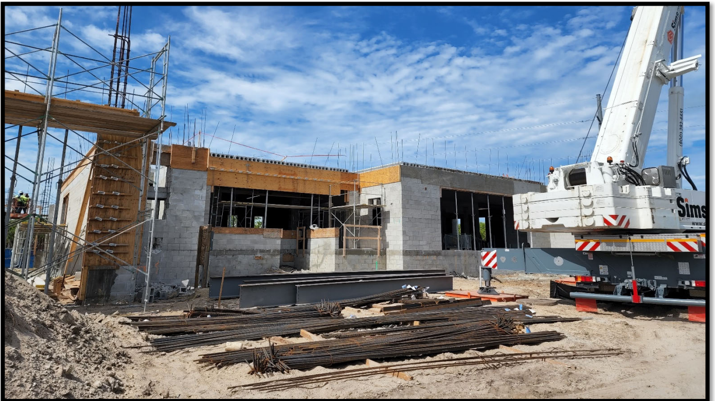
Fire Station 50 – Hollow Core Plank Installation and Framing for 2 nd Floor Slab
