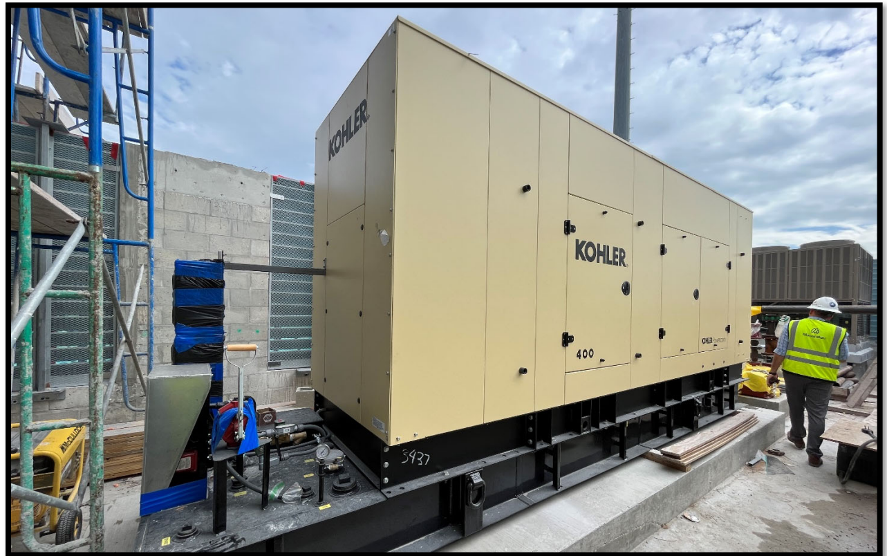
Fire Station 50 – Generator
