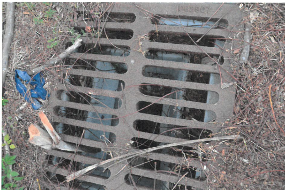
Figure 21: Storm drain insert becoming blocked with vegetative debris
