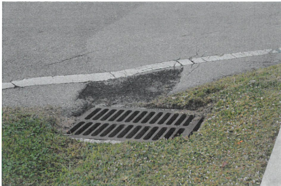
Figure 19: Road run-off directed immediately into stormwater grate
