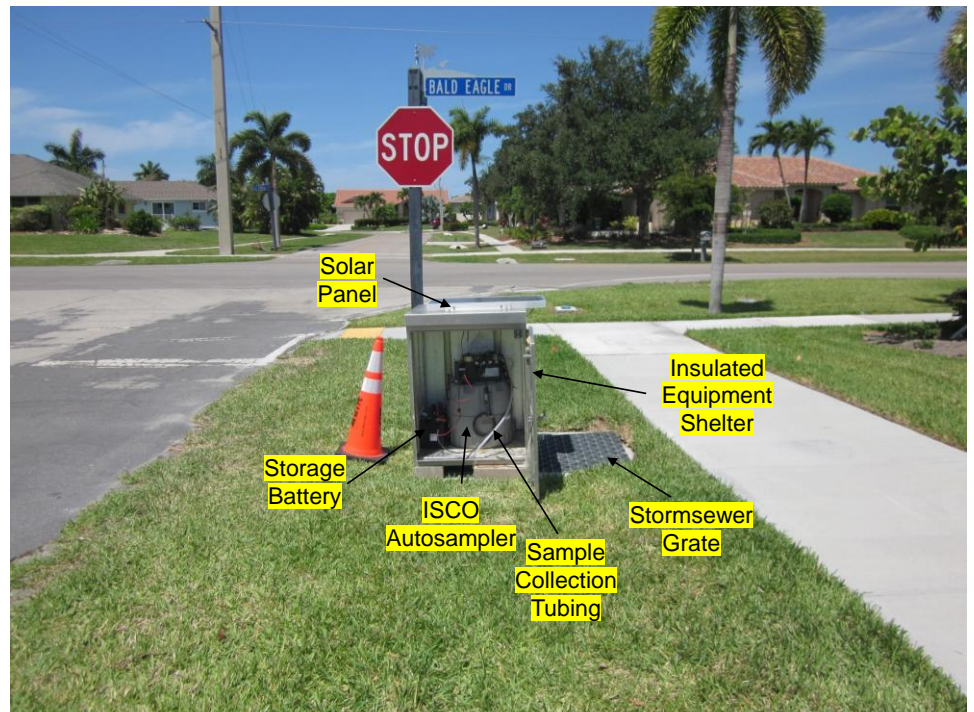
Figure 5-10. Photograph of Stormwater Monitoring Site MI-3. (Commercial watershed with partial reuse irrigation)
