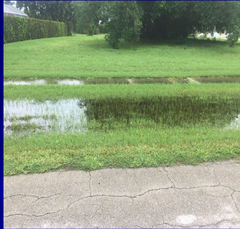
Swale system during storm events
